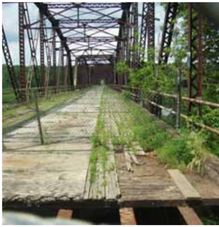
Decaying Long Meadow Lake bridge
