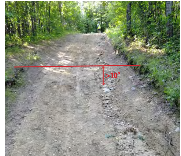
Severe Trail Erosion
