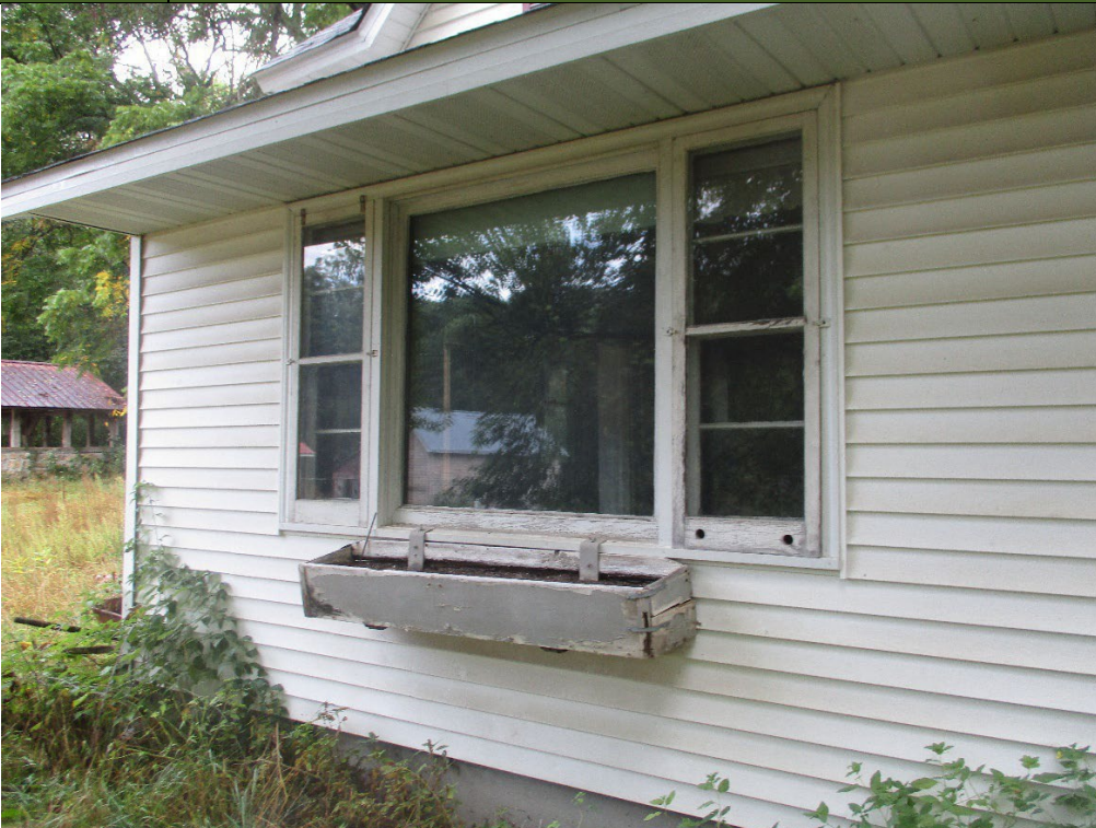
Photograph 2 09/03/26 Subject: Asbestos window glaze on west side of old house (3 panes)
