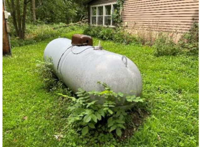
Propane tank located on the Property by the mobile home
