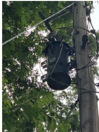
Pole mounted transformer located on the Property
