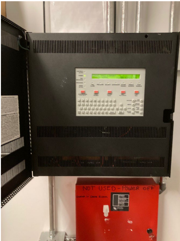
Figure 2 - Robert Trail Fire Panel
